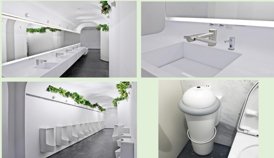
(Figure 13) Efficient quality of materials used in toilets and smart trash [19]
