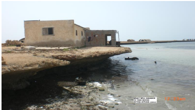
Fig. 5.5 Consequences of Coastal erosion in Dahlak Island
